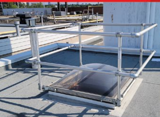
Guardrail for Skylight
