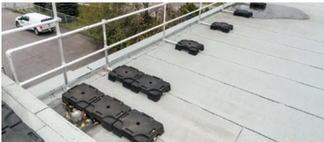
Roof drains - VSS Classic
