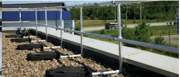
Ballasted roof - VSS Classic
